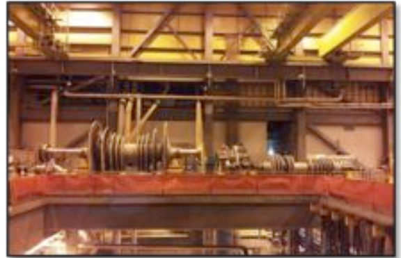
Unit 1 Turbine – Low-pressure section: and Intermediate and High Pressure section
